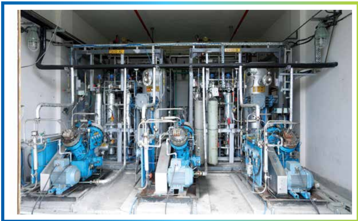
Hydrogen Generation Plant
