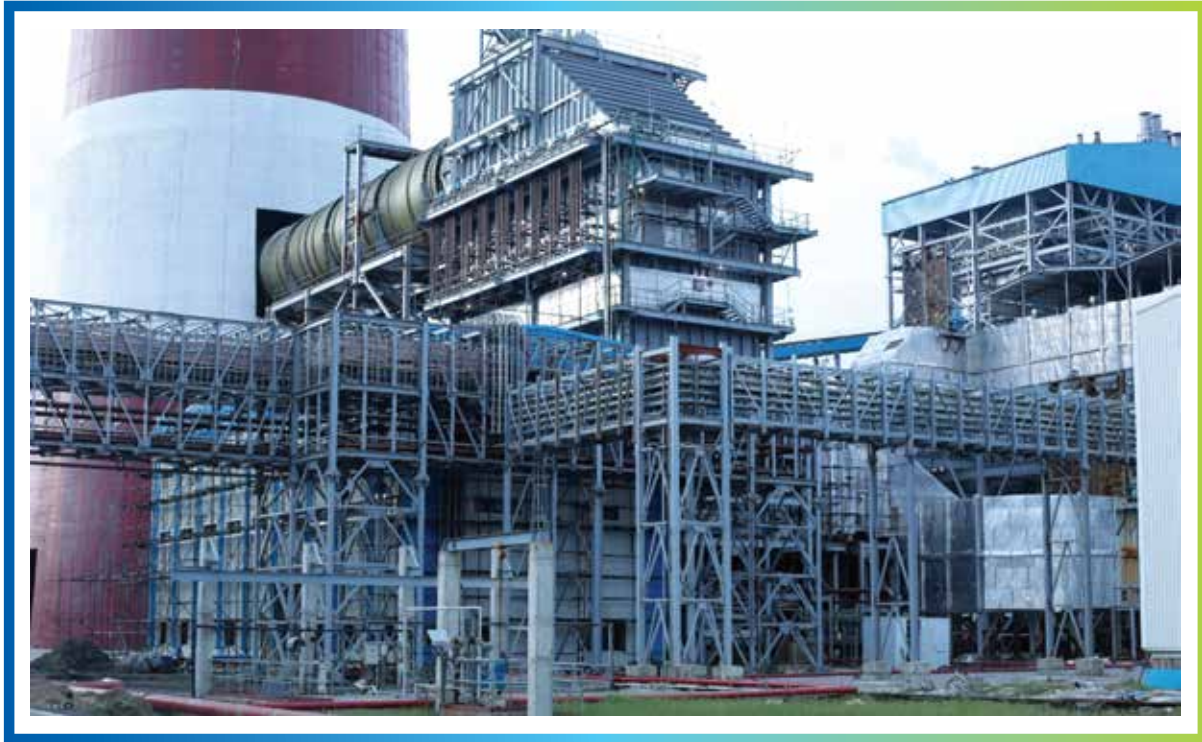
Flue Gas Desulfurization (FGD)
